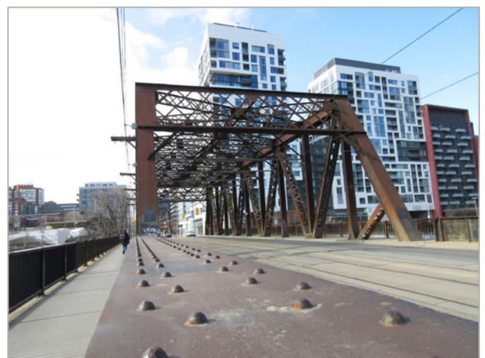
Sir Isaac Brock Bridge in a view looking north; the white condominium is on the site of the old Berg plant (see p.10). This steel structure was built in 1903 over the Humber River and moved here in 1916, when the streetcar tracks were added. The riveted surface is the top of a wall between the sidewalk and the traffic (it's visible across the street). Photo by the F&D
